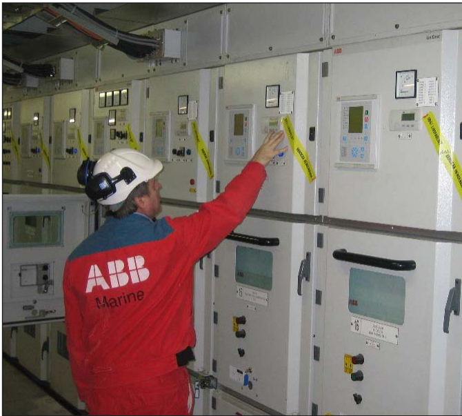
Picture 2: Medium-voltage switchgear monitored by fixed pyrometers
