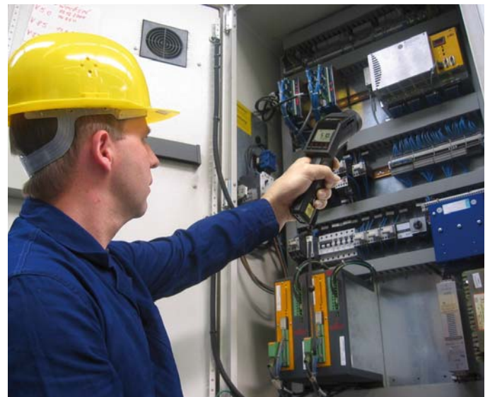
Picture 1: Temperature measurements on stressed components in a switch cabinet using the PSC LaserSight LS
